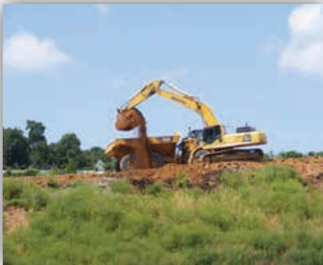
Jim Smith Contracting moving dirt on the I-24/I-69 ramp in Marshall County, KY.
