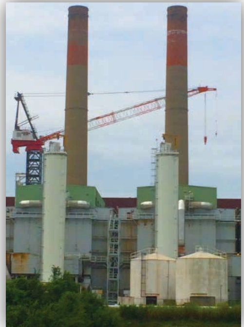
Pedestal crane at the Shawnee Steam Plant Scrubber project for AECOM Construction.
