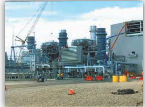
Combined Cycle Plant at the TVA Paradise Steam Plant in Muhlenberg County, KY.
